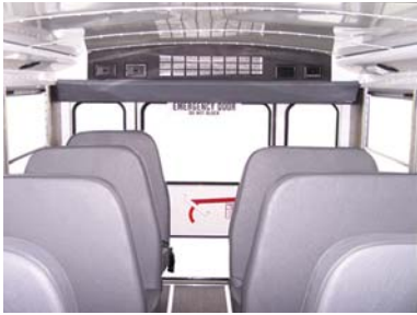
Wall Mounted A/C
